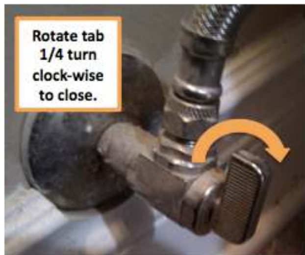
Kitchen or Bathroom
